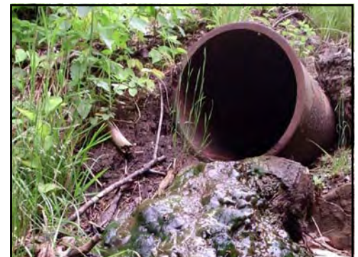
Ductile Iron Pipe (DIP)
