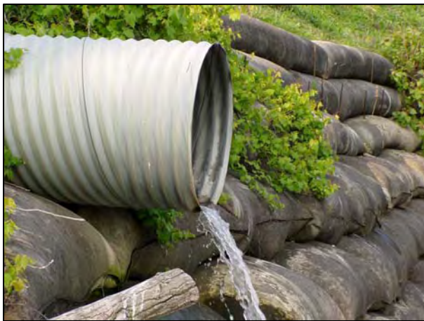
Figure 2: Storm Sewer MS4 outfall
