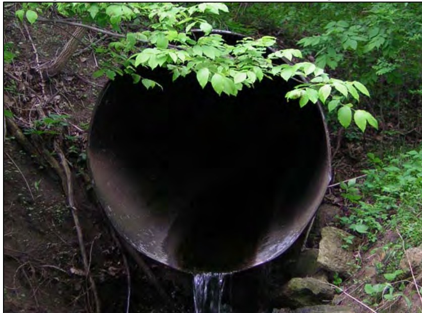
Figure 11: MS4 outfall location with illicit discharge
